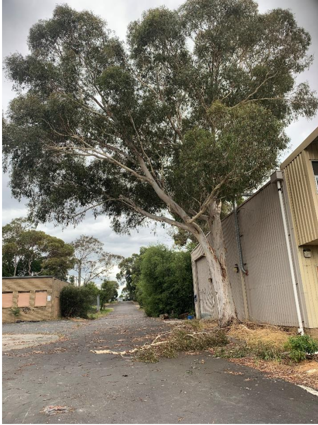
Tree 111 - recently fractured branch lying on the road.
