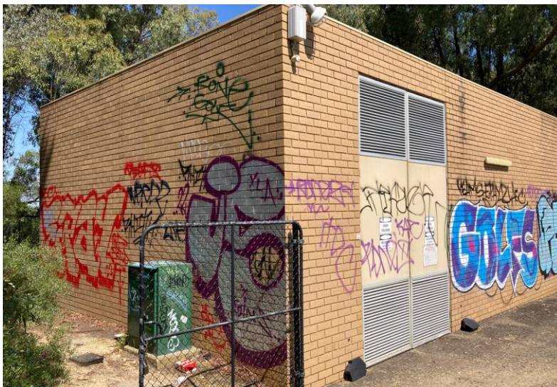
Figure 3 Substation – western side ventilation grilles
