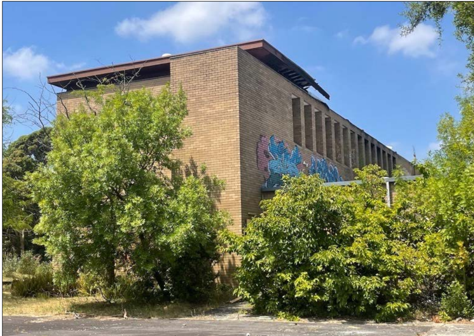
Figure 8 The Administration Building viewed from the west. Note roof partially destroyed by fire.
