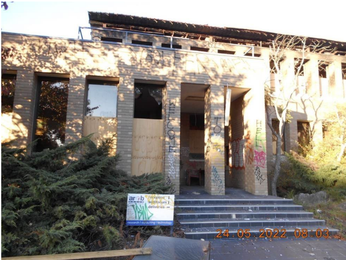
Figure 9 – Damage to the exterior of the main building
