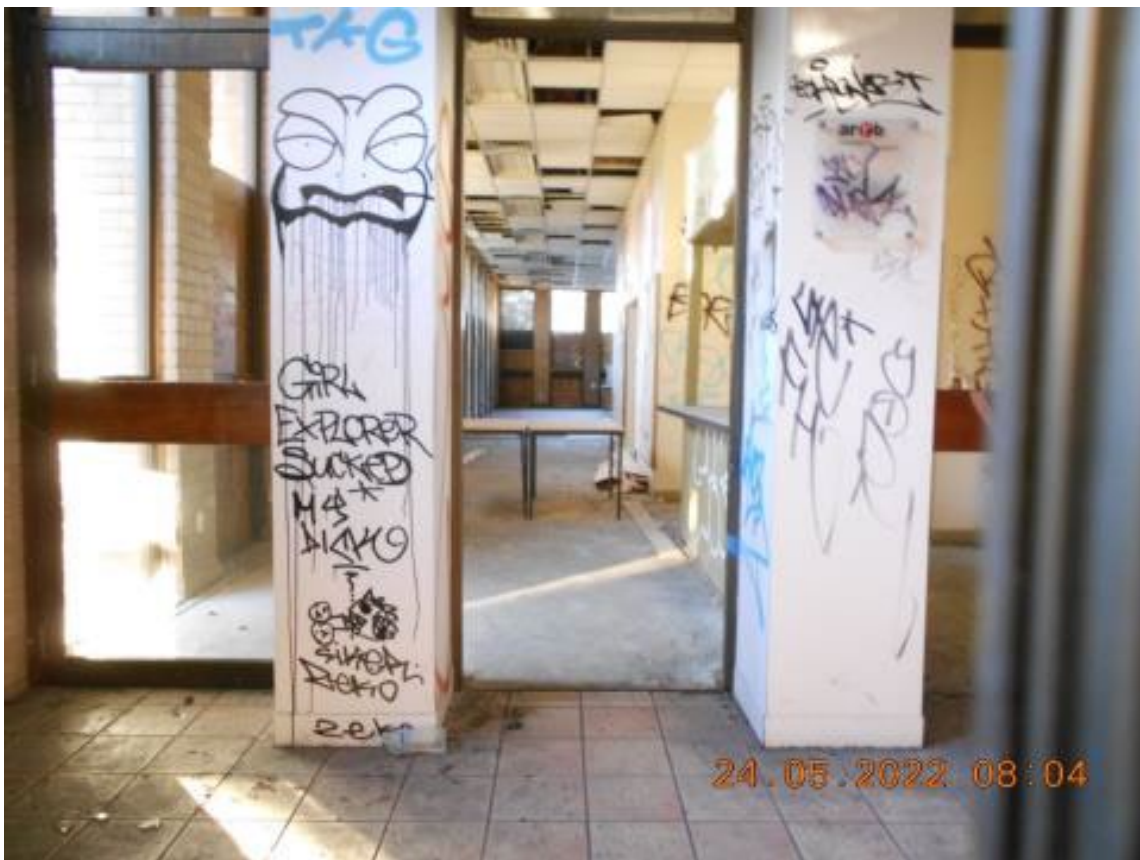
Figure 10 - Graffiti damage to the inside of the main building
