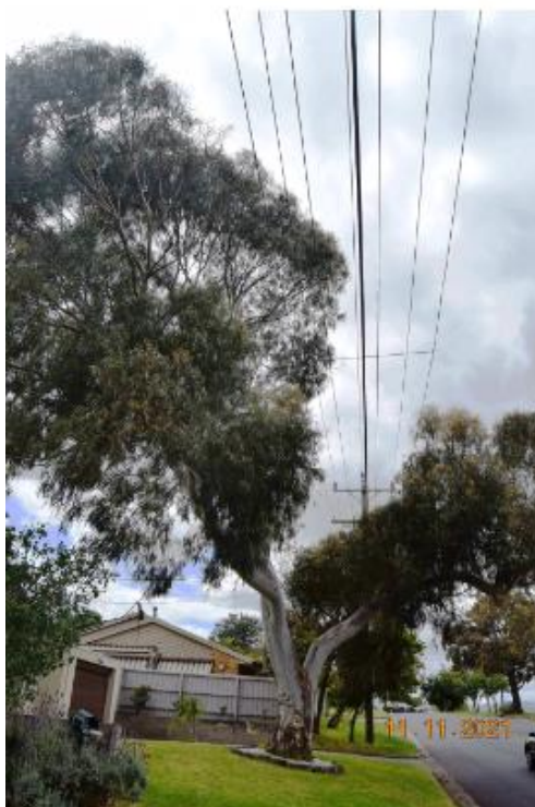
Figure 4 Street tree in conflict with electric lines
