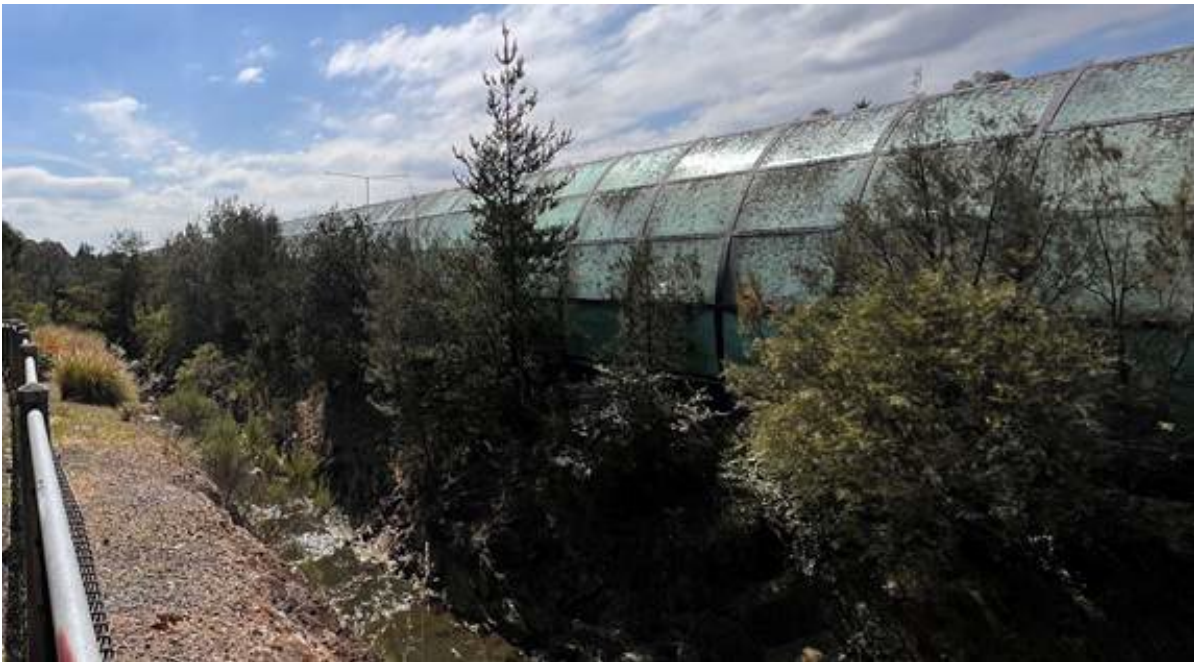
Example of compromised transparency in acrylic noise walls further west along Eastern Freeway (now demolished)
