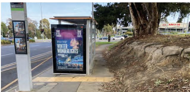
Figure 37 Springvale Road narrow footpath due to erosion and effecting DDA accessibility
